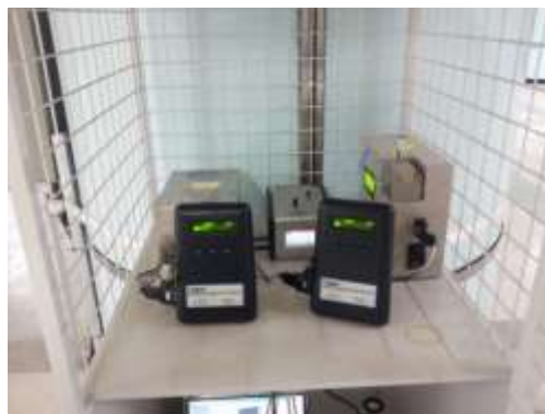
Figure 1. The PM measuring instrument Airtest PM2500 installed at a subway station
