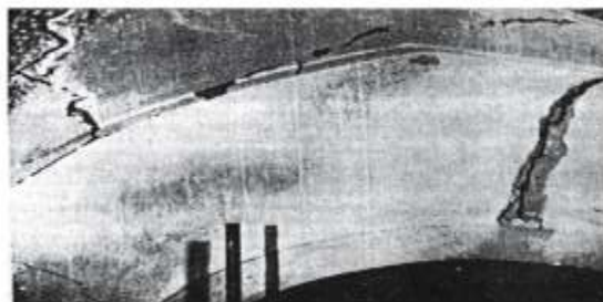
Fig. 1. Vibration caused crack of an old church near road [4].
